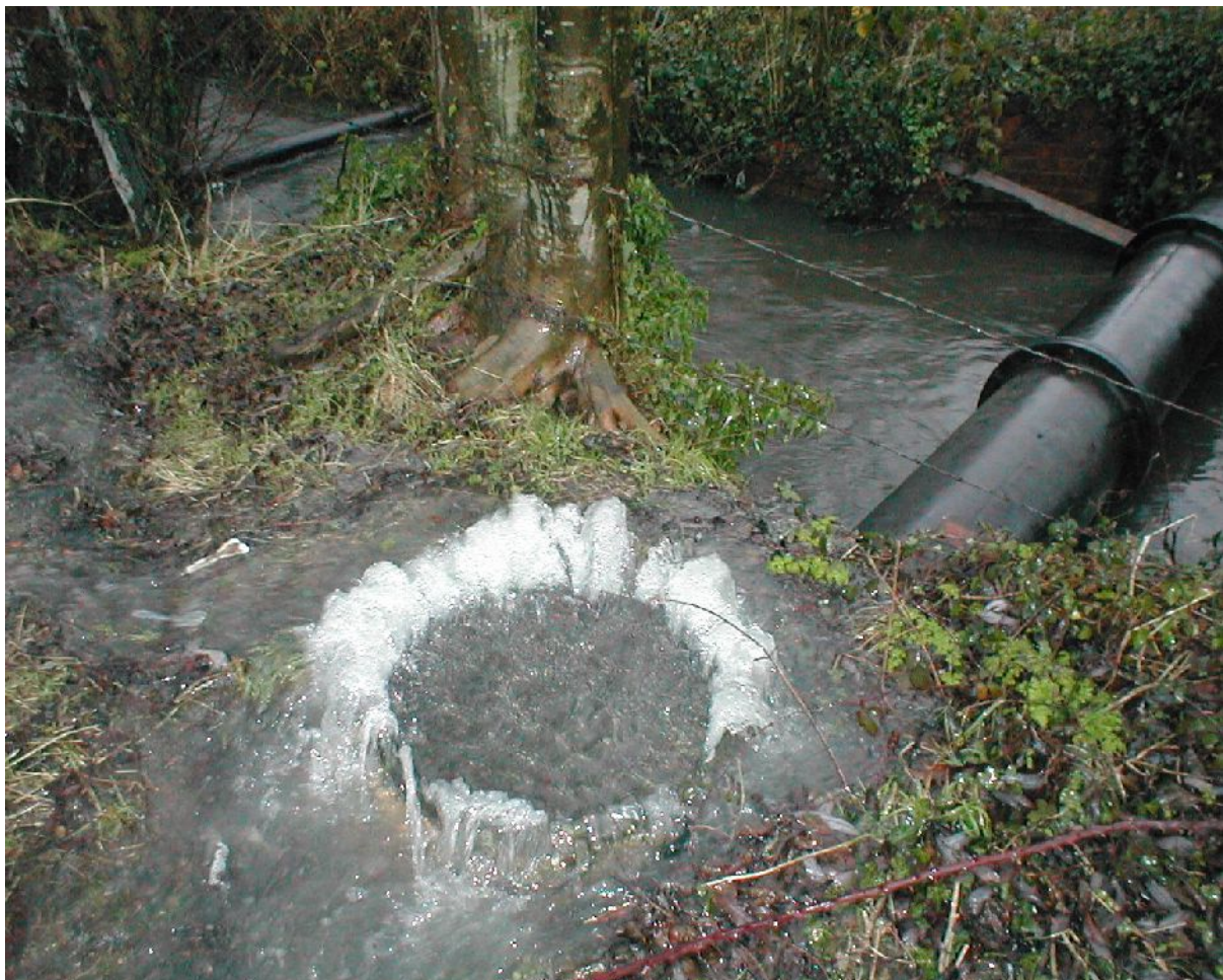
Sewer surcharging during moderate rainfall, Bridgend (Water 21)
