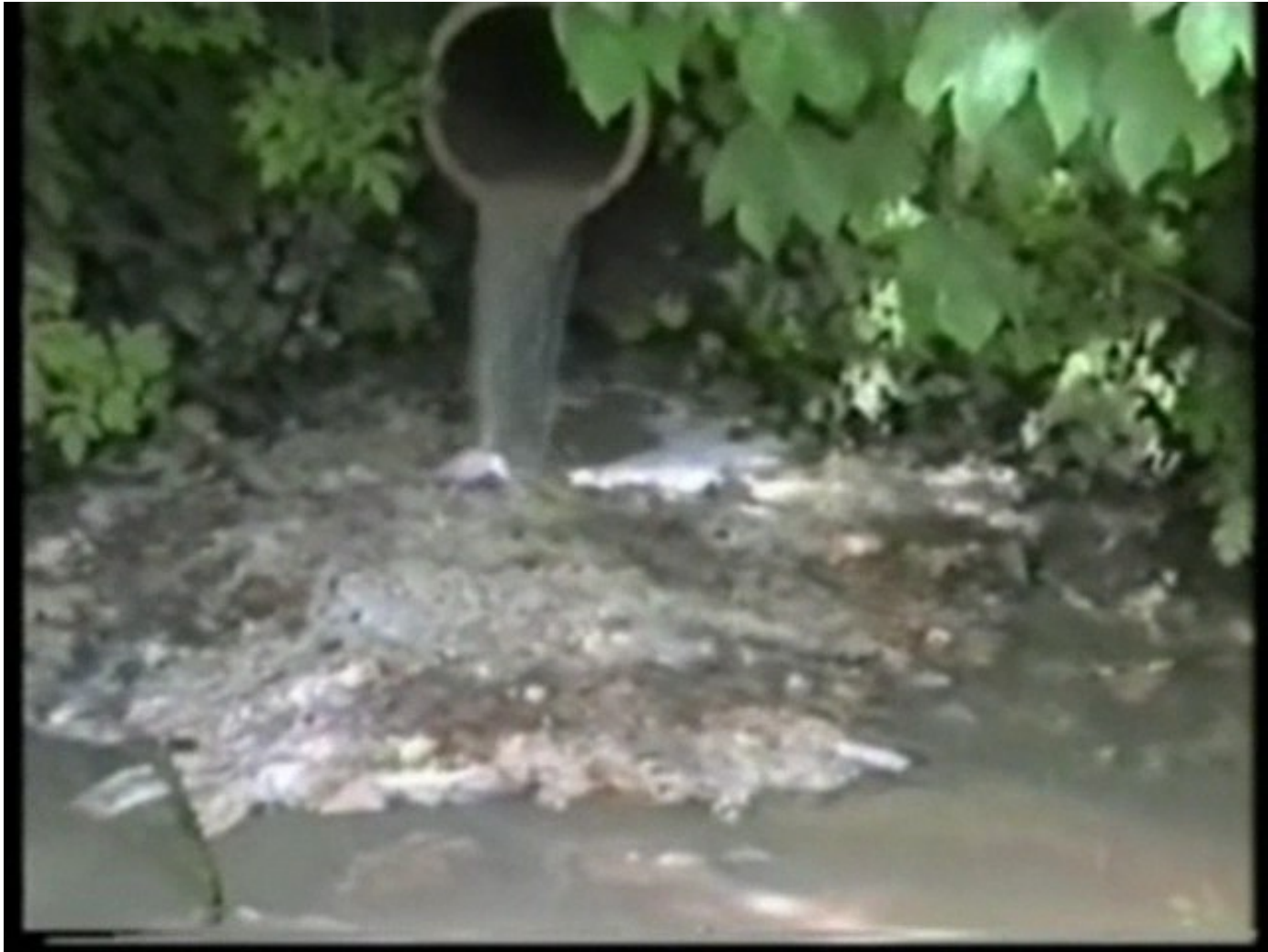
Still from video, storm overflow operation
