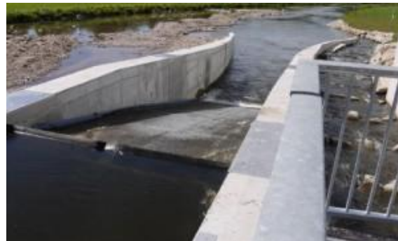
The Enclosed Kaplan unit installed between the channel walls
